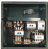
Interior View of MU-G20W FASD
