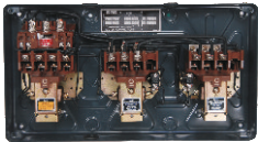
Interior View of MK2 SASD
