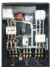
Interior View of MU-G30W FASD
