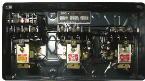
Interior View of MK1 SASD
